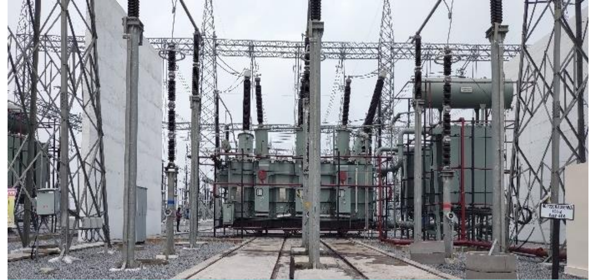
APTransCo./03 : 315 MVA Power Transformer at 400/220 KV SS Rachagunneri
