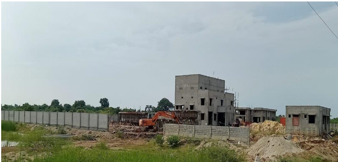
APIIC-04 : 10MLD Water Treatment Plant
